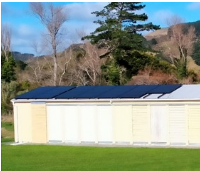
The test building housing the hot water systems under investigation on a sunny winter's day. Three of the hot water systems are connected to the solar photovoltaic panels on the roof
